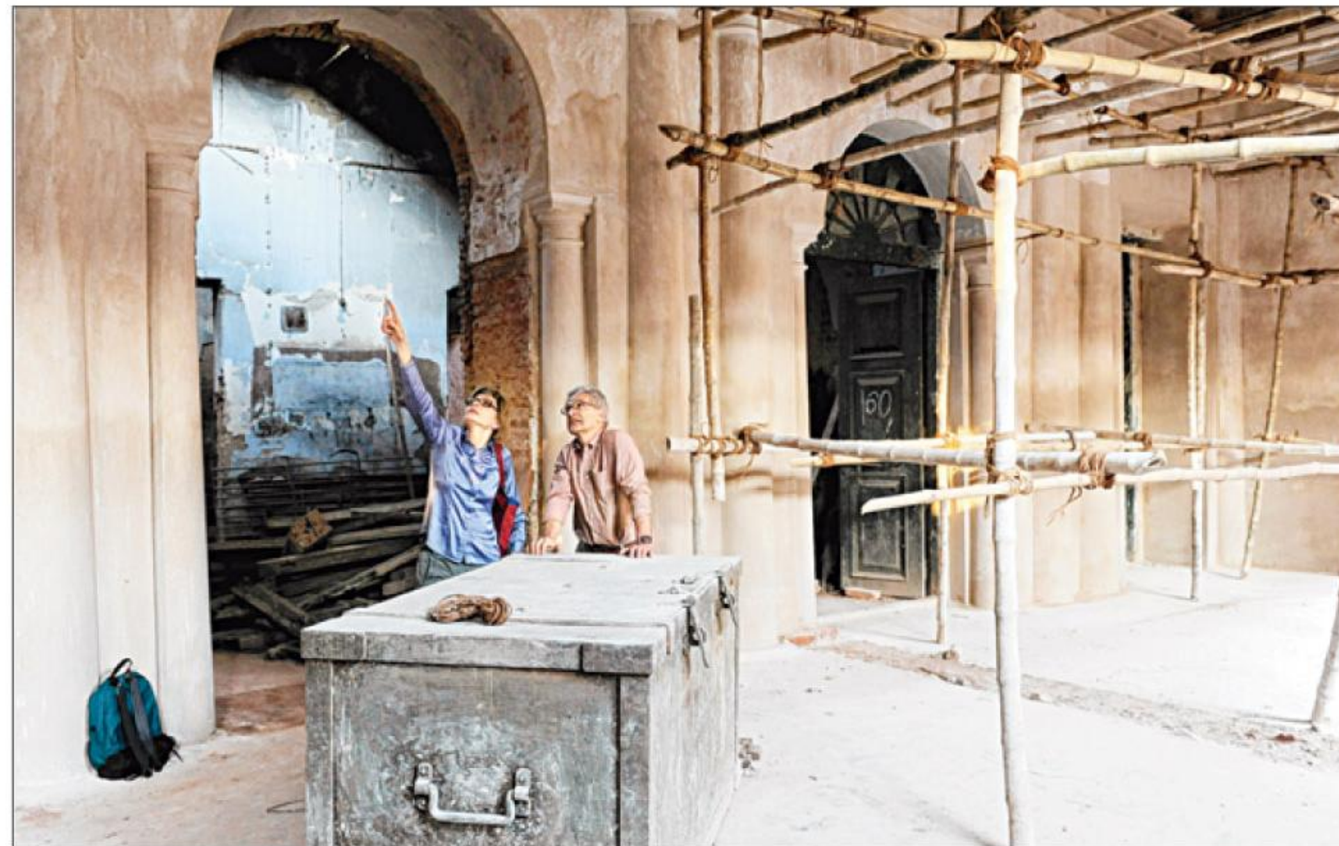
Bente Wolff, curator, National Museum of Denmark, and (right) architect Flemming Aalund check out the restoration work being done at the former Danish Government House. Pictures by Pradip Sanyal
